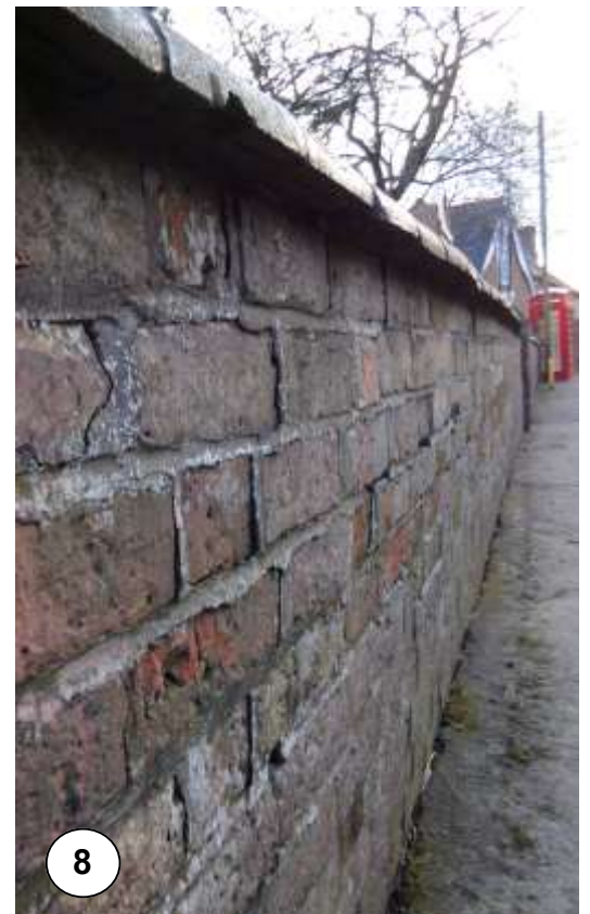
Figure 8. Spalling mortar and irregular brickwork
