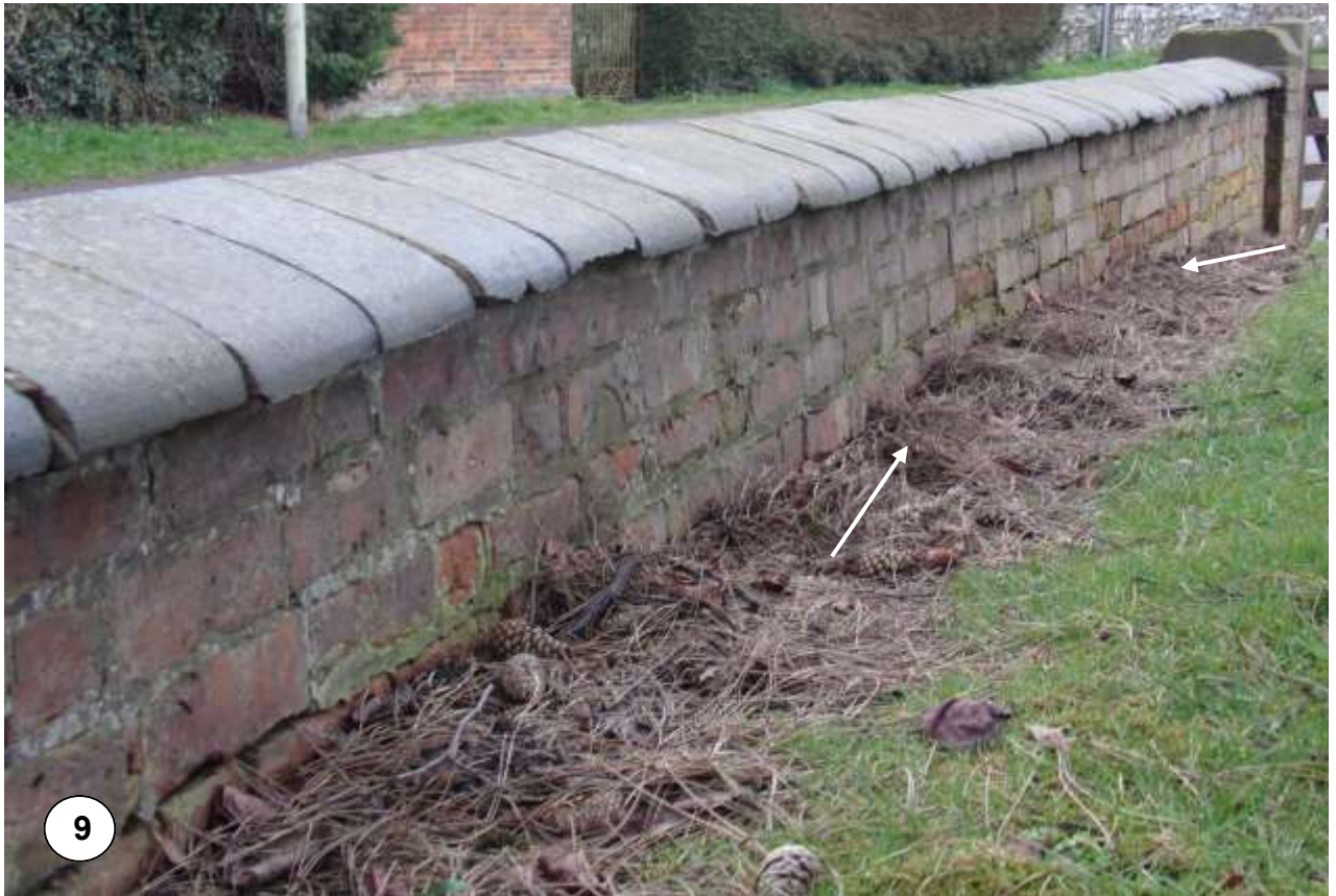
Figure 9. Churchyard side of wall. Curvature of bulge is clearly visible between the arrows. Note absence of mortar in brickwork at ground level at bottom left.
