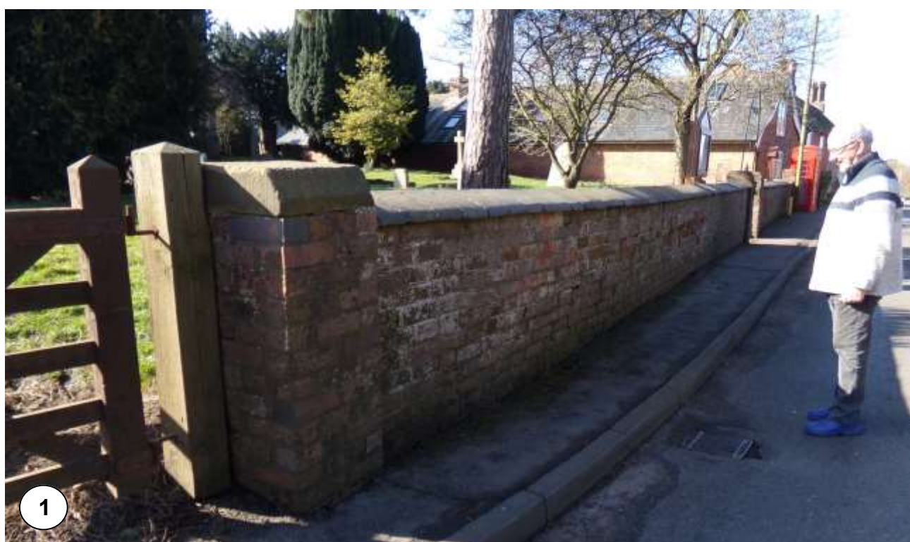
Figure 1. Eastern end of churchyard retaining wall. The bulging area is in front of the standing figure.
