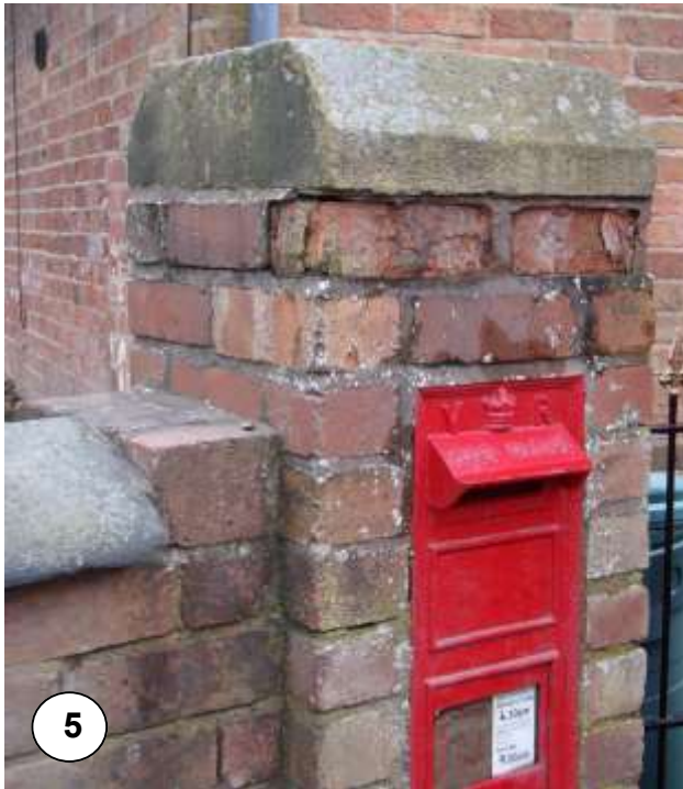
Figure 5. Spalled bricks above the letter box
