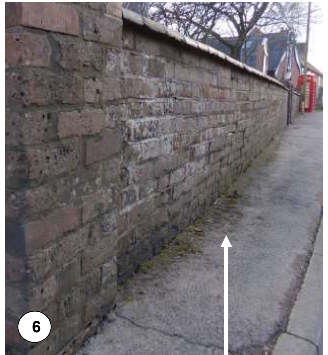
Figure 6. Location of bulge near eastern end of wall
